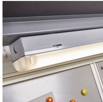
LED light with above bench light rail
